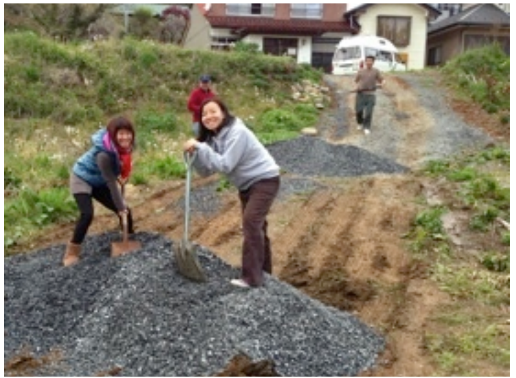
Filling the mud slope outside Ahn Sensei's home with gravel so that cars can be driven up.
